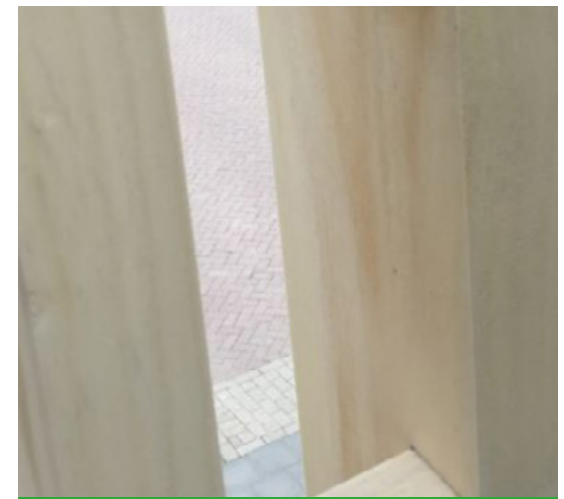
8.5 Reddish brown staining
