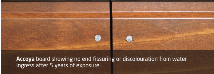
Western red cedar board showing end-grain disfigurement from water ingress after 5 years of exposure. Note also coating detachment along shoulder detail.
