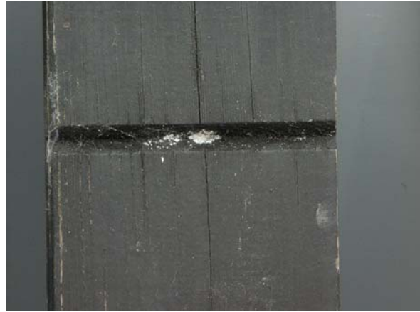
Wood cracks in acetylated Scots pine finished with an opaque black acrylic coating after 9½ years outdoor exposure (sample 25001).
