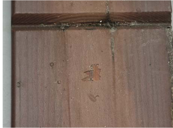
Cracking of coating surface (sample 12003) as result of coating degradation after 9½ years of outdoor exposure.
