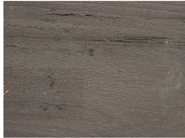
Cracking of coating surface (sample 21004) as result of coating degradation after 9½ years of outdoor exposure.
